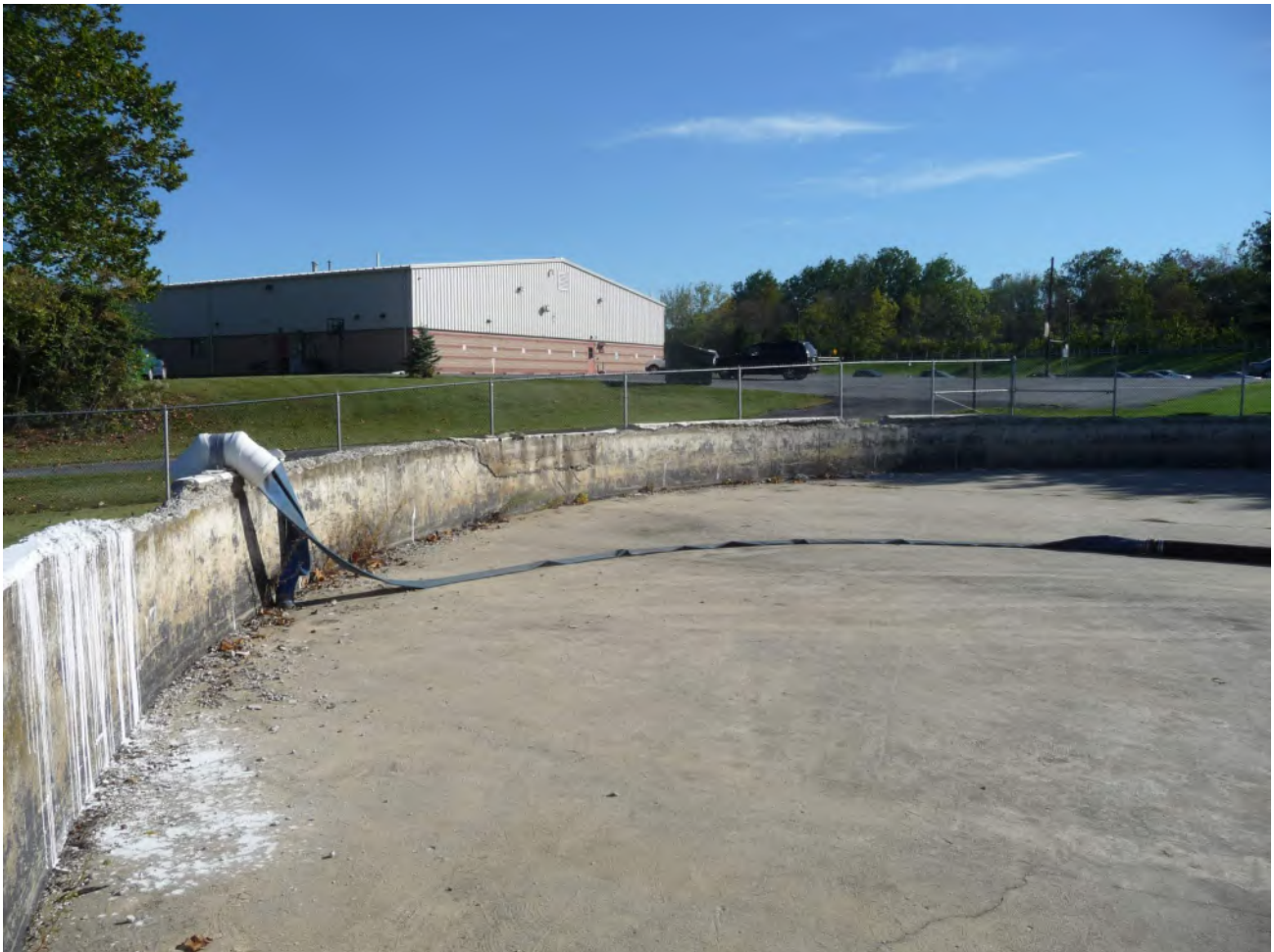
Picture 13: Abandoned Bio-Reactor Tank
