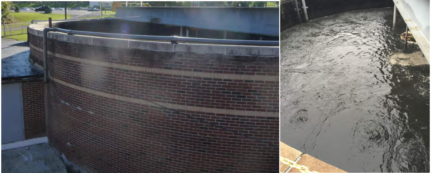
Picture 18: Large Sludge Holding Tank
