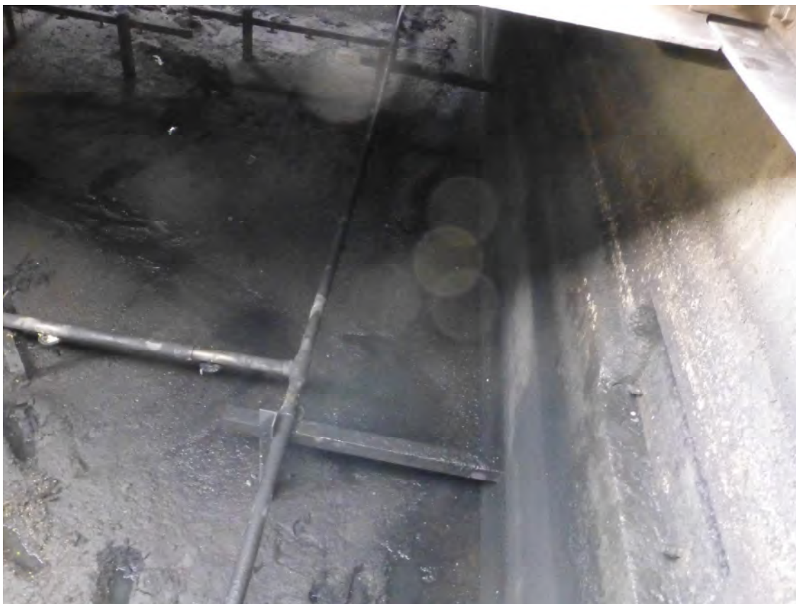
Picture 7: Accumulated Grit in Pre-Aeration Basin
