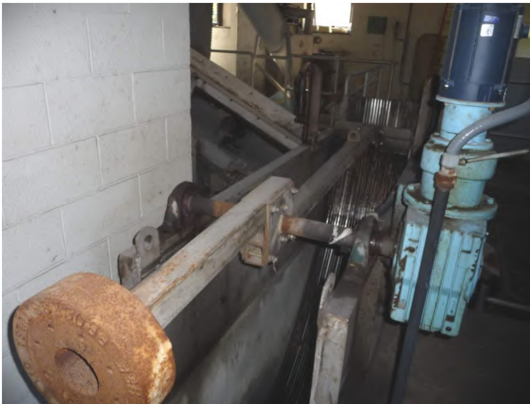
Picture 5: Bar Screen with Mechanical Arm
