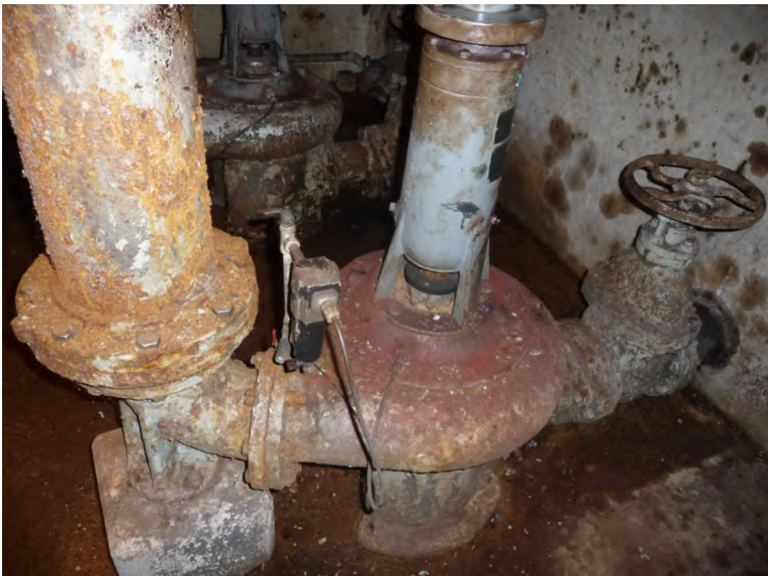
Picture 1: Main Pump Station Pumps
