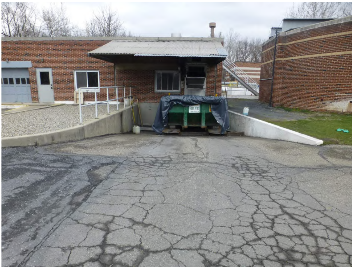
Picture 22: Sloped Pavement in Front of Dumpster
