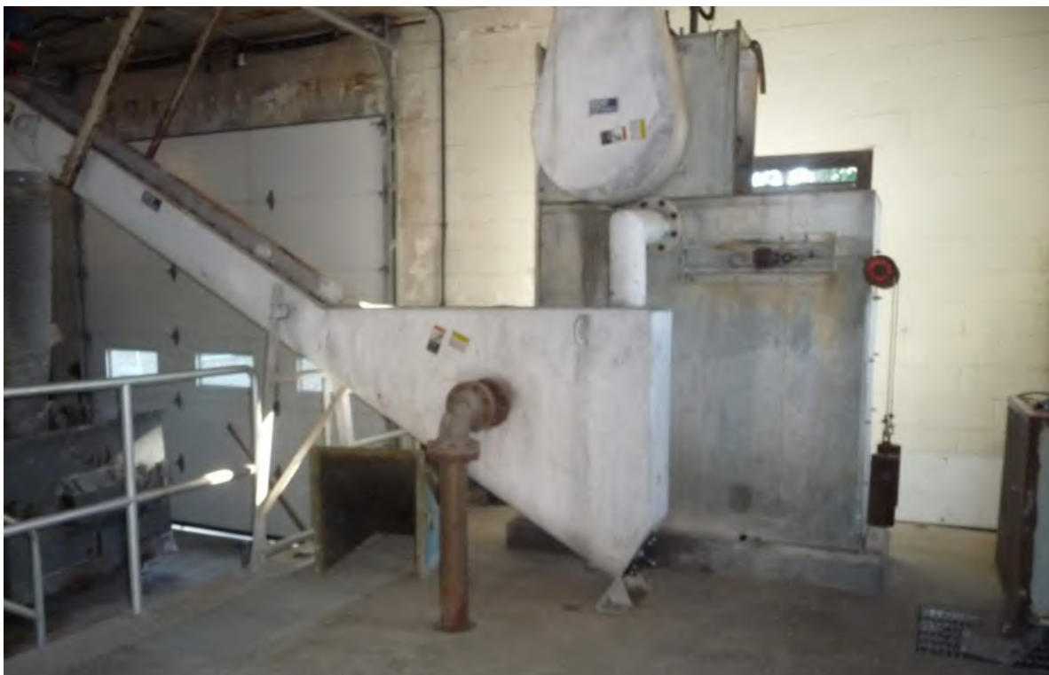
Picture 6: Grit System: Bucket Elevator and Dewatering Screw
