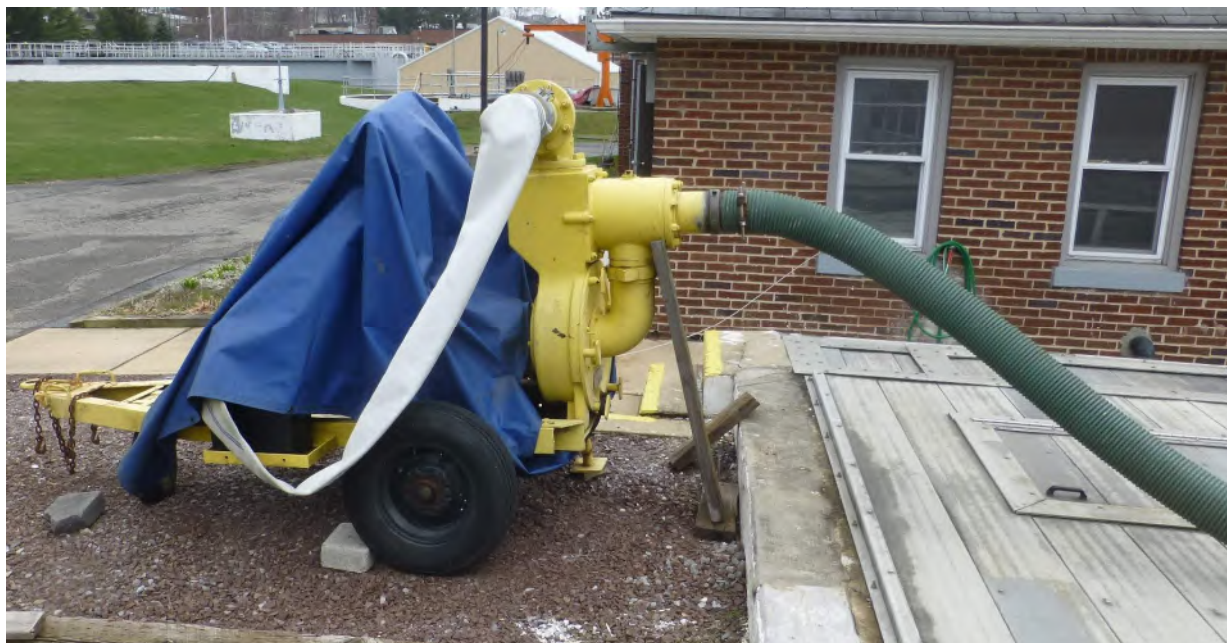
Picture 11: Portable Pump Used to Supplement Primary Lift Station
