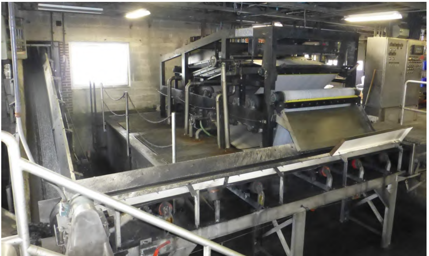
Picture 20: Belt Filter Press with Conveyor System
